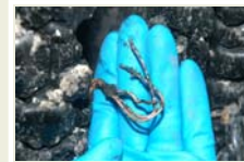
Suspect electrical wiring discovered during an investigation
